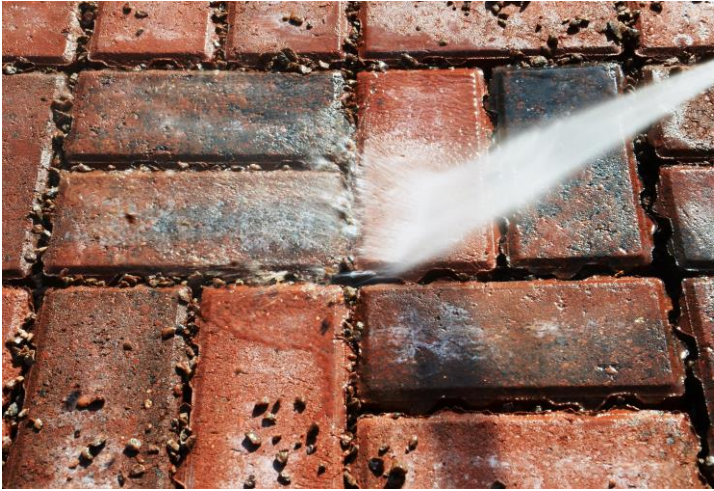
Jointing aggregate readily dislodged from maintenance regimes to unclog voids
