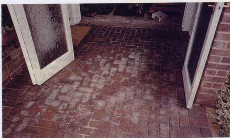
Figure 1: The unsightly effects of efflorescence on a domestic driveway/path.
