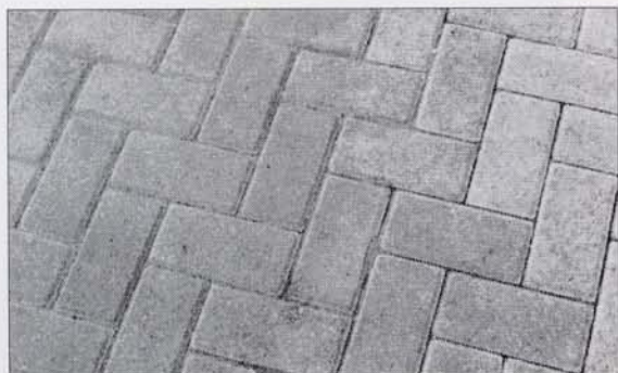
Figure 2. Aircraft Pavement Partially Treated with Polymer
