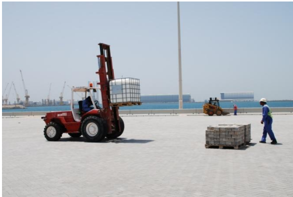
Resiblock 22WB in 1000 litre IBC are place on site at relevant intervals.
